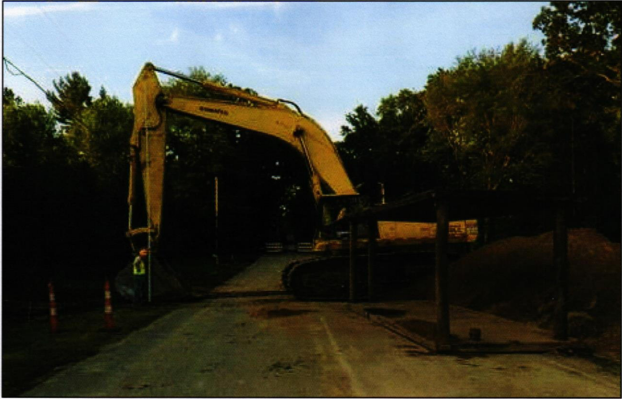
A 25' long grade rod is being held up to the excavator arm. During excavation, a 35' clearance is required to maintain a safe distance of 10 feet from any power lines.
